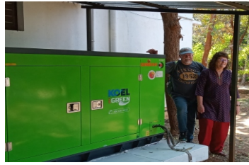
Mr. Jon & Ms. Jennifer Dietz, USA at the Generator they donated to Pravaham, 18 th Feb. 2023
